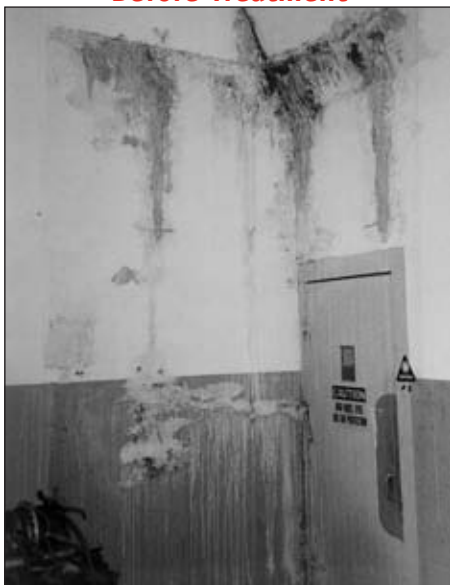
Hydrostatic weeping just below the Electric House.
